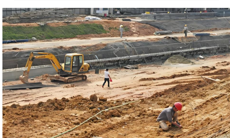
Construction emergency power
